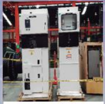
Medida Interior e Interruptor Sm6, Nexans Colombia
