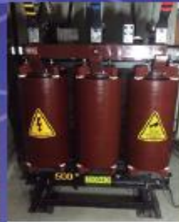
Transformador resina, Impact Print S.A.S
